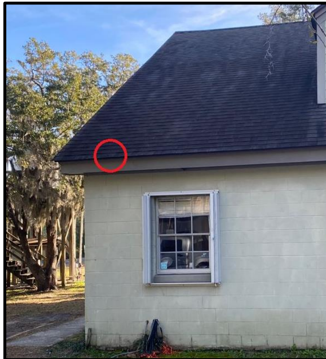
Photograph 14. ACM-14 – Roof shingle hanging over western exterior wall.
