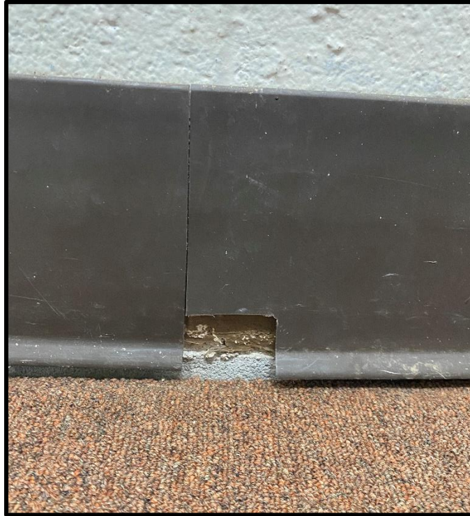
Photograph 7. ACM-7 – Baseboard on northern wall of Office 1.
