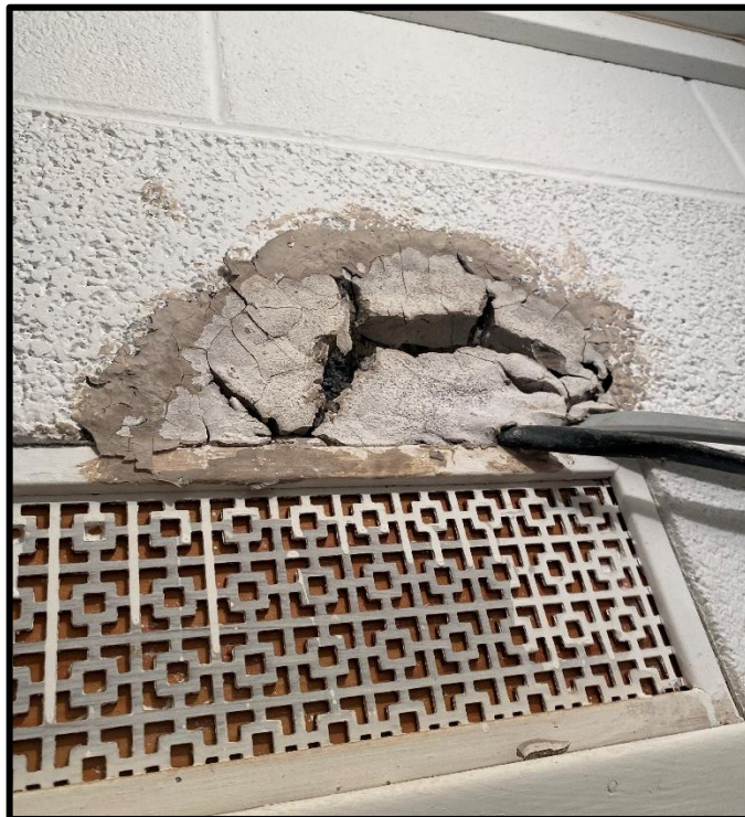
Photograph 6. ACM-6 – Wall material above doorway in Office 2 Closet.
