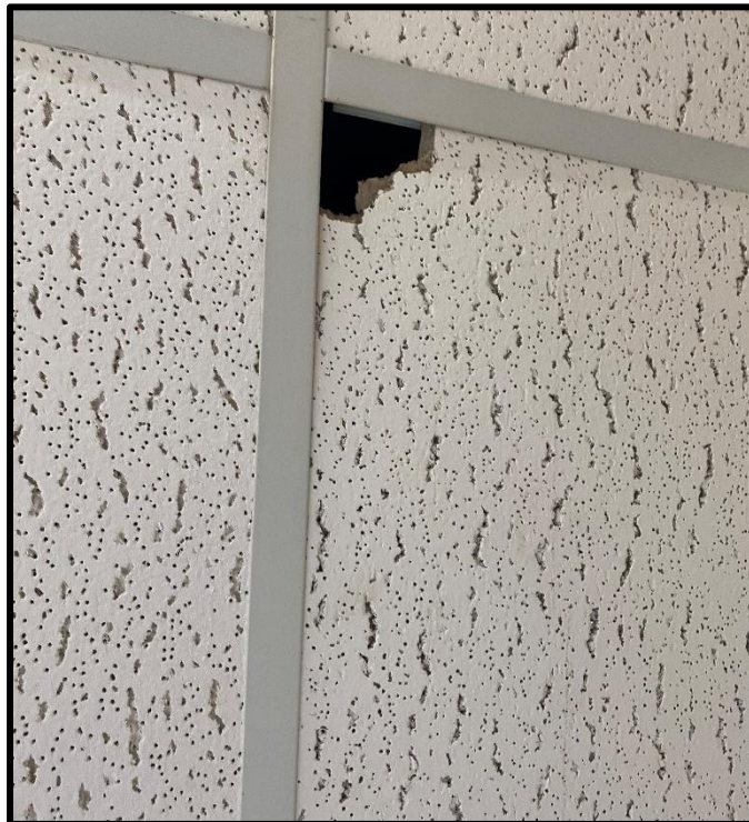
Photograph 2. ACM-2 – Ceiling tile in northern portion of Break Room.
