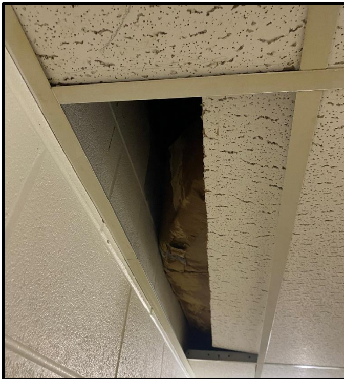
Photograph 4. ACM-4 – Ceiling tile near western wall of central Corridor.
