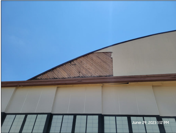
SECTION OF WALL DAMAGED FROM STORM
