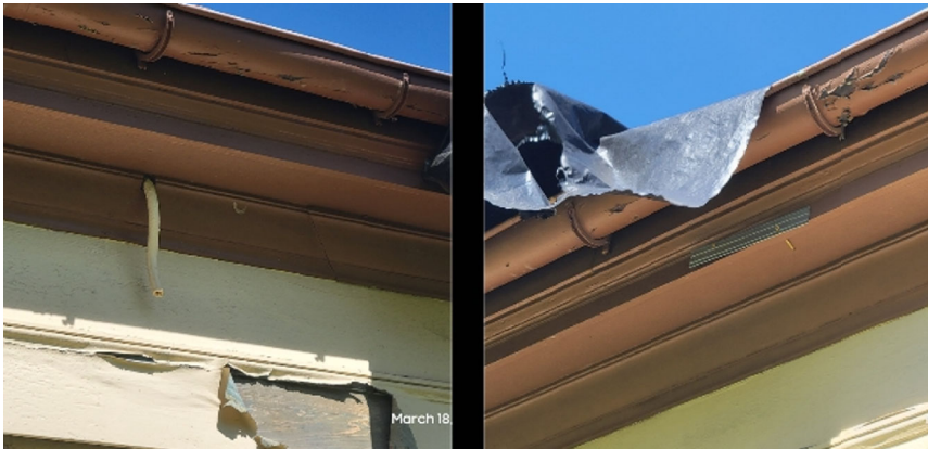
EXAMPLES OF SOFFIT, FASCIA, TRIM CONDITIONS.
