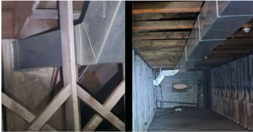
CURRENT HVAC FRESH AIR INTAKE.
