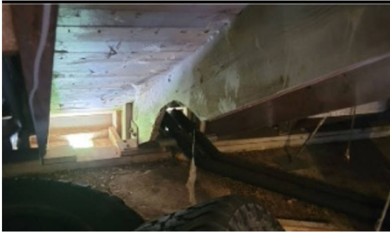
EXAMPLE OF RAFTER TO BE REPAIRED
