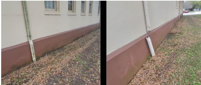
EXAMPLES OF DOWNSPOUT CONDITIONS.
