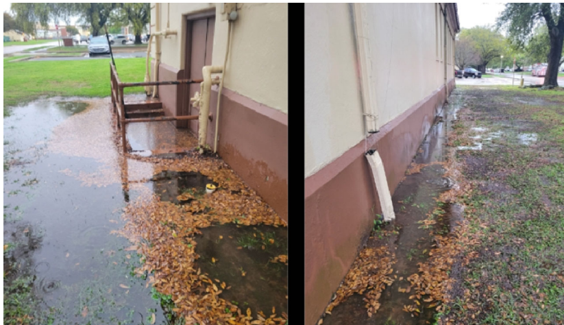
EXAMPLE OF CONDITION AFTER RAIN
