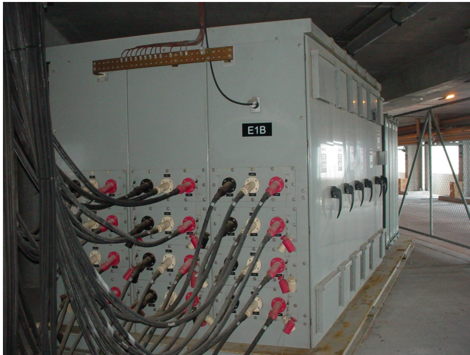
Figure 12-6. Double-Deck Pier Switchgear
