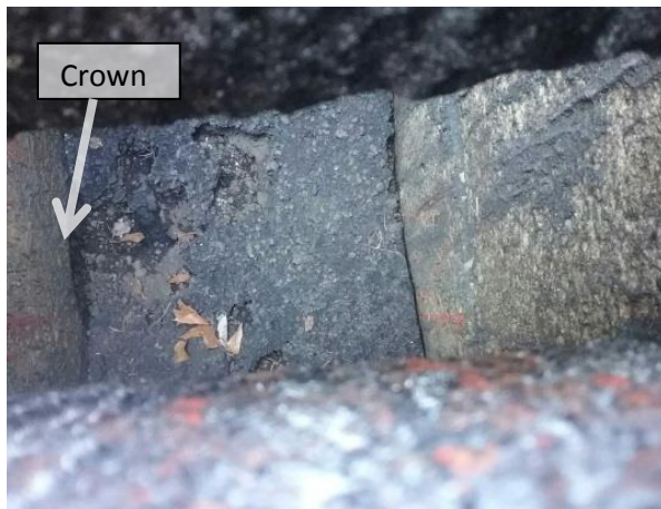
Figure 21: Inlet Full of Asphalt to Pipe Crown
