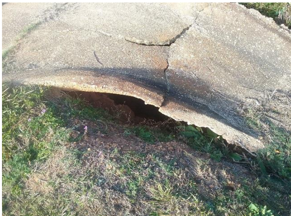
Figure 35: Cracked Flume with Erosion
