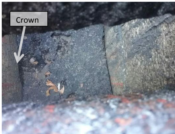
Figure 21: Inlet Full of Asphalt to Pipe Crown
